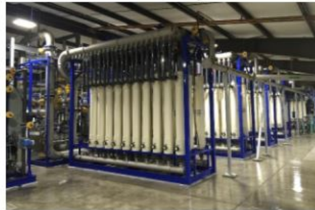
Advanced Water Treatment Facility
